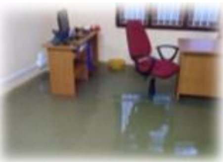
Offices used by our partners have flooded causing difficulties in the day to day management of our projects.
